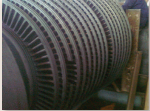
Picture 2: Damage to Barring Gear
